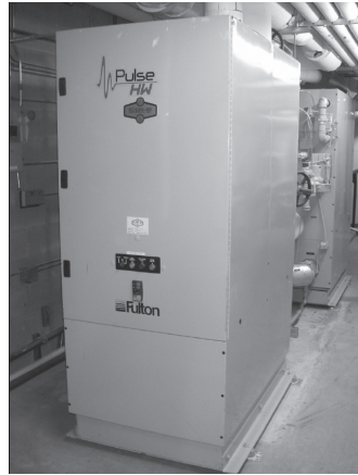
(2) New Boilers. Photograph by Steve Rubbert.
